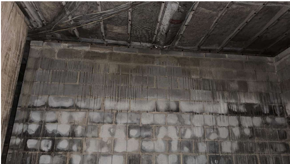
FIGURE 6: CRAWLSPACE MOISTURE DRIVE
