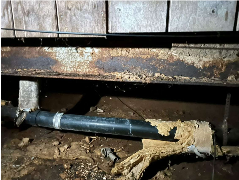
FIGURE 7: STRUCTURAL SUPPORT AND CRAWLSPACE DEGRADATION
