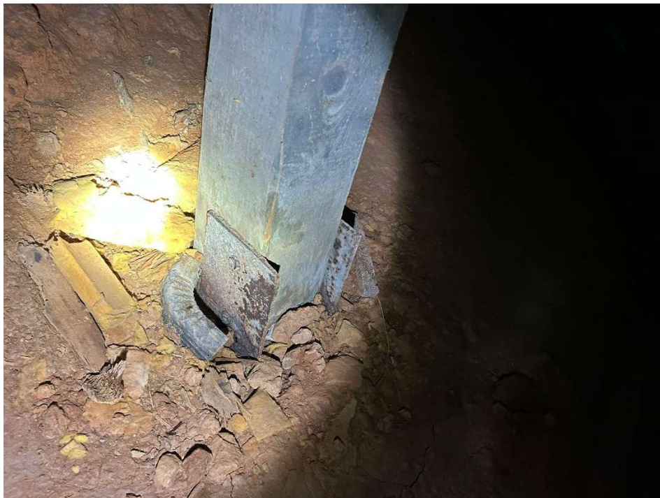
FIGURE 4: ISOLATED SUPPORT DEFICIENCIES
