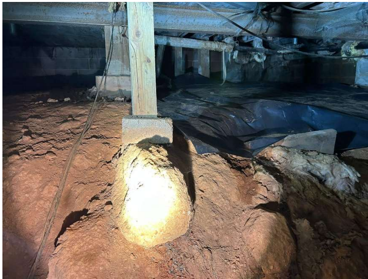
FIGURE 8: SAGGING GIRDERS IN CRAWLSPACE DUE TO LACK OF POST SUPPORT
