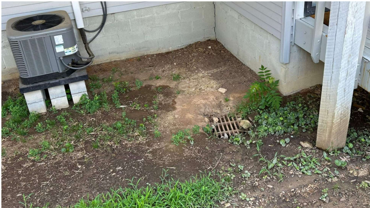
FIGURE 5: DRAINAGE ISSUES AND FOUNDATION DETERIORATION
